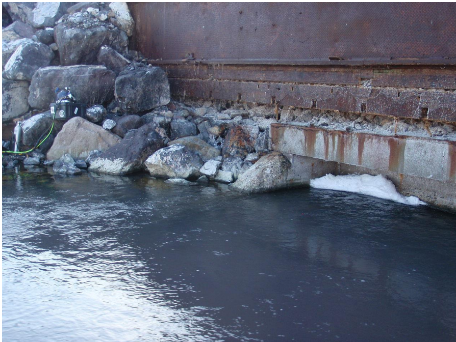
Photo 2-View of North Side of East Culvert. The water level is approximately 1.5 to 2 feet lower than in March 2013
