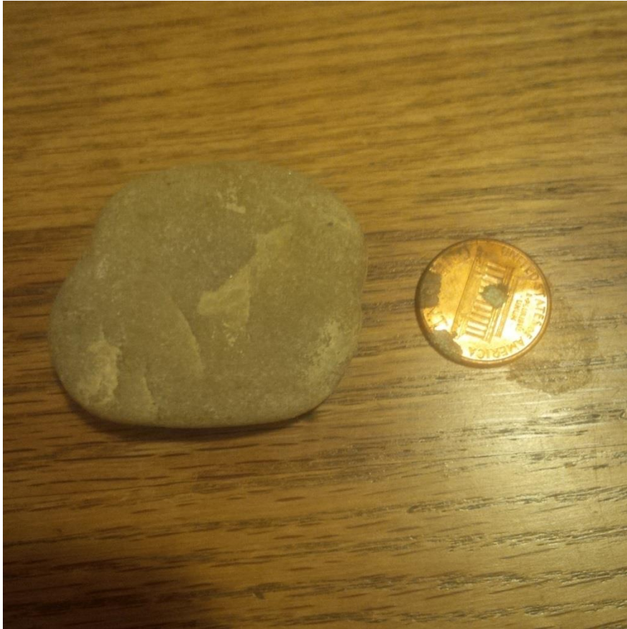
Photo 1- Sample of rounded rock taken from pile at base of crack in the west sidewall of the East Culvert. This is presumed to be original backfill material.
